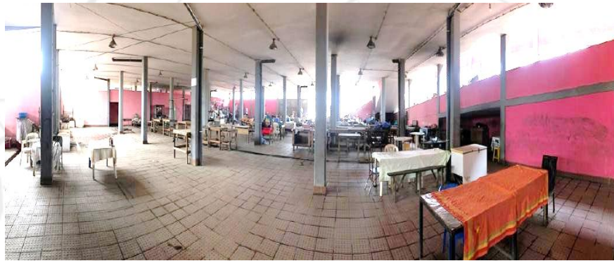
FIG 26: INTERIOR OF MERCADO DA CHAPADA. MOST TRADERS ABANDONED THE SPACE AND ARE TRADING ON SIDEWALKS NEARBY.
