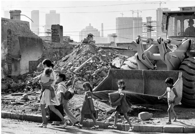
FIG. 46: DEMOLITION IN PROGRESS, DISTRICT SIX, CAPE TOWN, CIRCA 1974-1975. TAKEN DURING THE FINAL STAGE OF REMOVAL OF 6 000 FAMILIES FROM DISTRICT SIX, FOR RELOCATION TO THE CAPE FLATS AND ATLANTIS, IN TERMS OF THE GROUP AREAS ACT.
