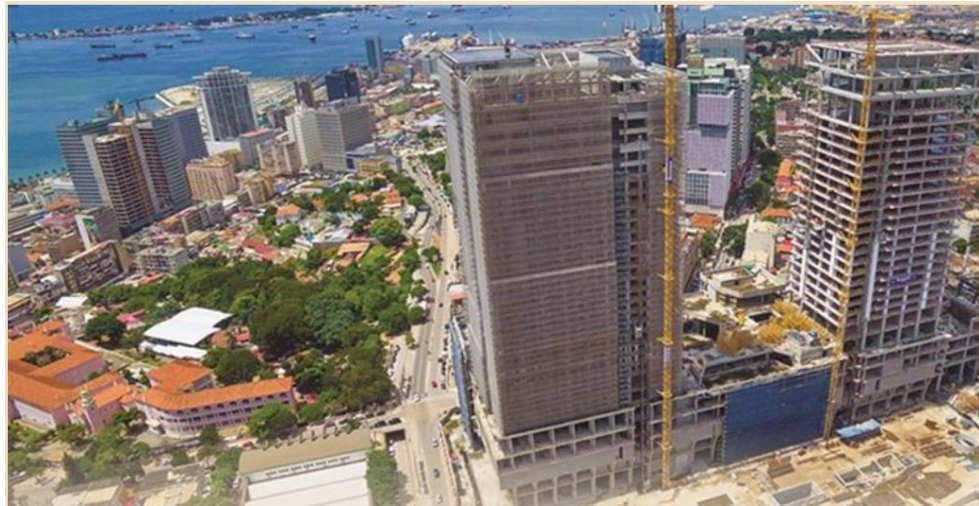
FIG 29: THE ONGOING CONSTRUCTION SITE OF KINAXIXI MULTI-USE COMPLEX SOURCE: https://expansao.co.ao/angola/interior/faltam-500-milhoes-usd-para-acabar-as-obras-do-kinaxixi-111930.html (ACCESSED: 14 JANUARY 2024).
